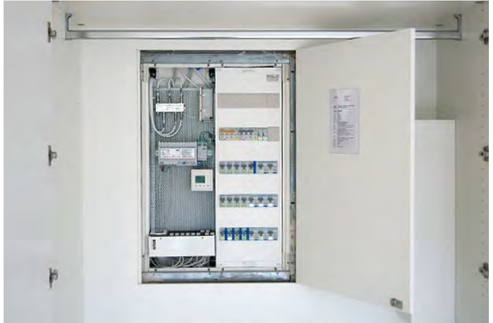
Fuse box (in each apartment)
